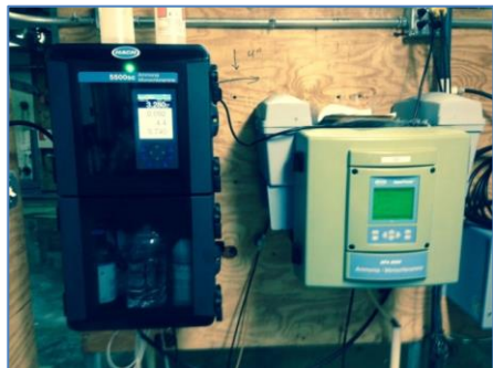
Figure 2A: Hach process instrumentation measuring finished water prior to entering the distribution system
