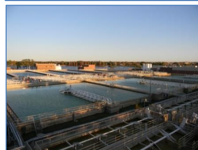
Figure 1: Bachman WTP test facility in Dallas, TX
